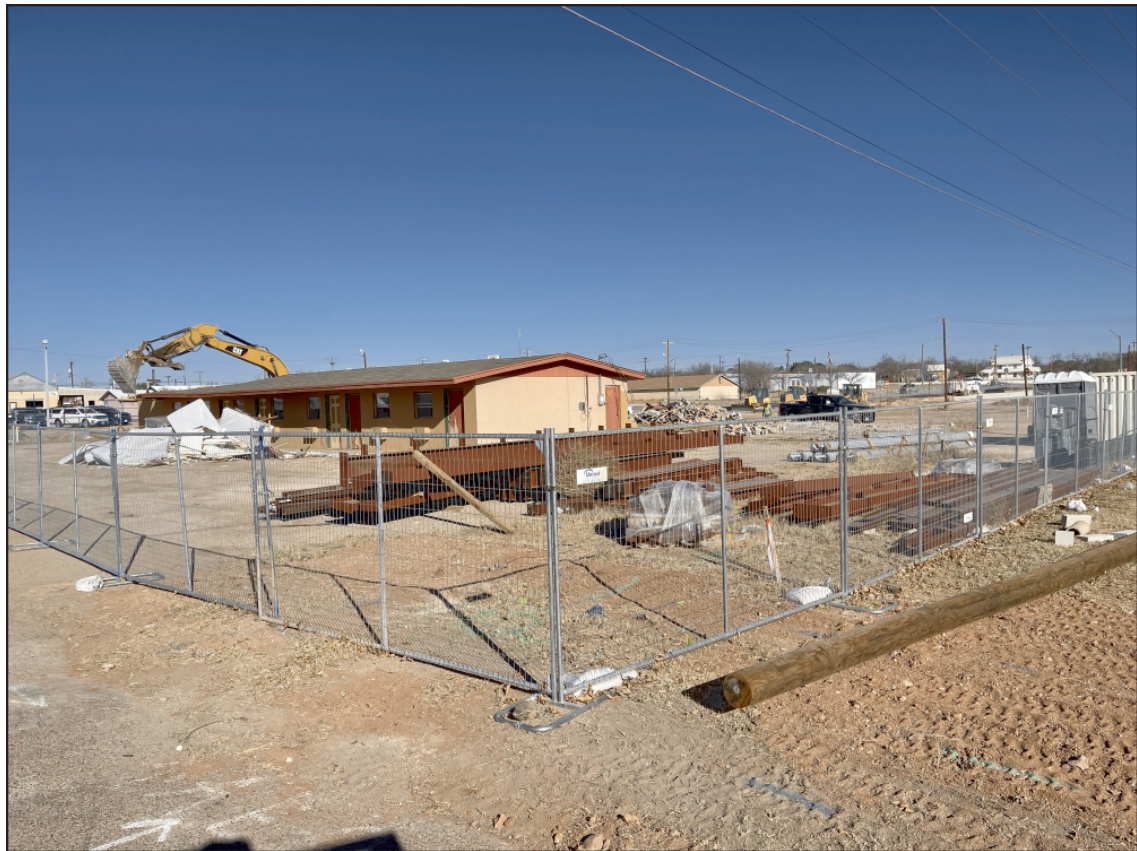
Progress! Demolition was underway last week on the old Mountain Creek Lodge in Robert Lee. The motel is being torn down to make way for a new convenience store.
