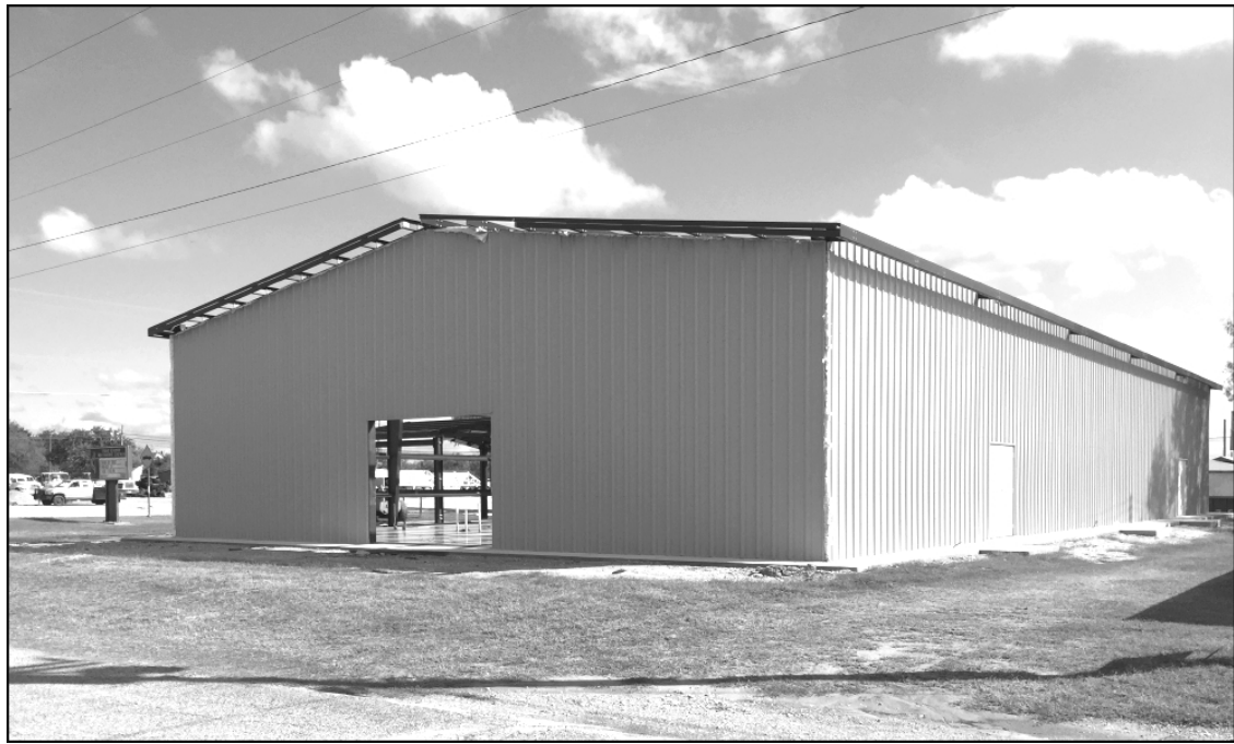
Coming Right Along! The new building for Robert Lee's First United Methodist Church is beginning to take shape. The church is constructing the building to be used by the congregation, and also by the community of Robert Lee.
