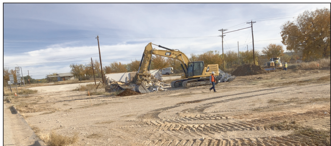
Demolition! Things are in the works to make way for the new convenience store in Robert Lee. A street between Highways 158 and 208 has been closed and the old Friendship Cafe building has been demolished in preparation for the new store. There is also a construction fence up around the old motel in advance of its demolition.
