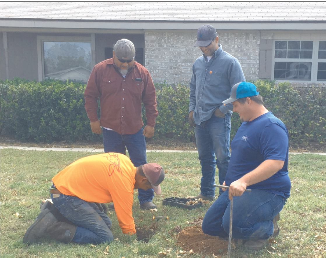
New Meters! Robert Lee city workers and others worked in yards and alleys replacing the old water meters with new digital meters. The new program is the result of a 70/30 grant received by the City of Robert Lee for this purpose.
