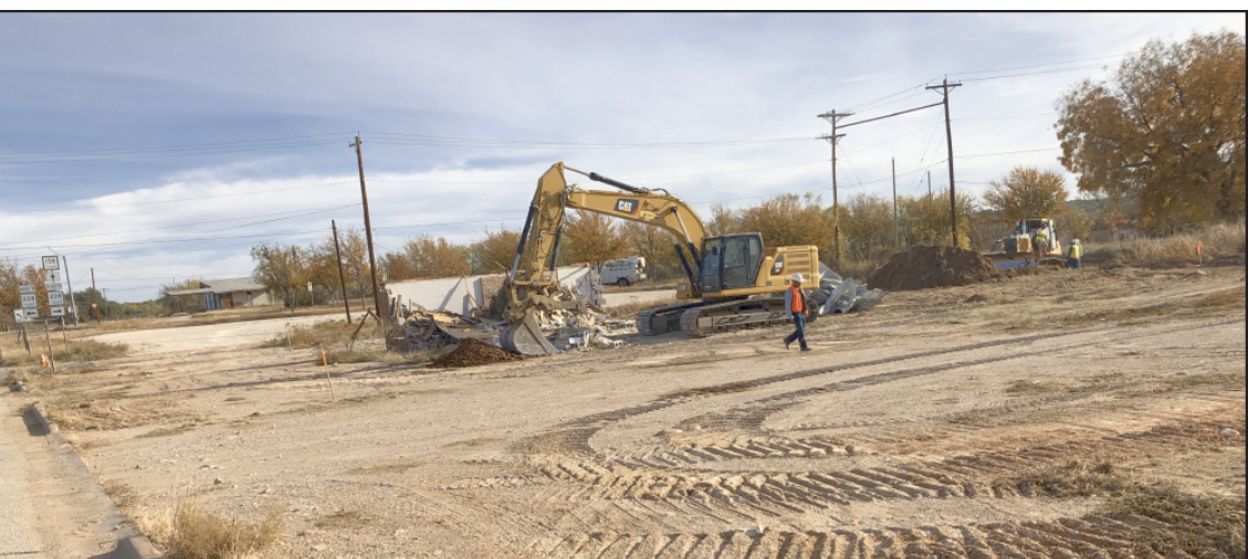
Demolition of restaurant buildings, the old motel and even a street make way for the new convenience store at the Hwy 208/Hwy 158 intersection in Robert Lee
