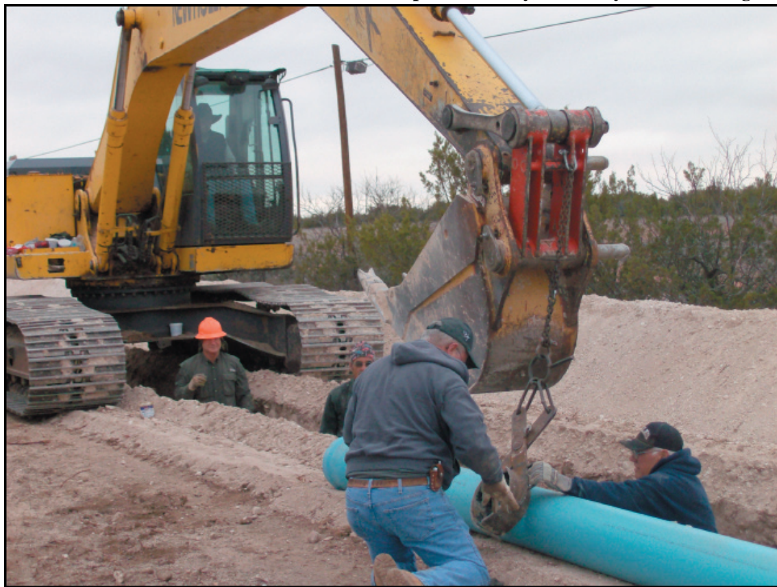
Robert Lee Pipeline! Tommy Shook operates the excavator while (from left) Marshall Millican, Charles York, Joe David Key, and Jerry Horn work to make the connection for the water pipeline from Robert Lee to Bronte.
