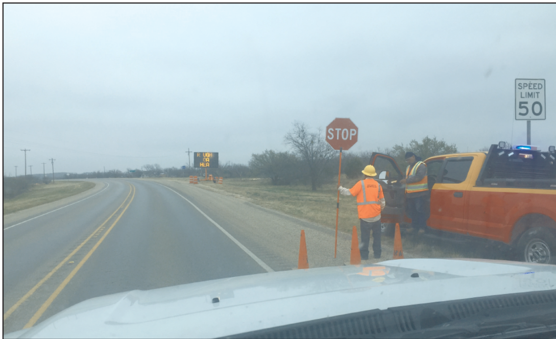
And so it has begun! The road construction, originally scheduled to begin on January 21, 2019, has finally started on Highway 277, north of Bronte. Traffic was stopped at the Kickapoo Creek bridge at the north edge of Bronte on Monday afternoon, March 11.
