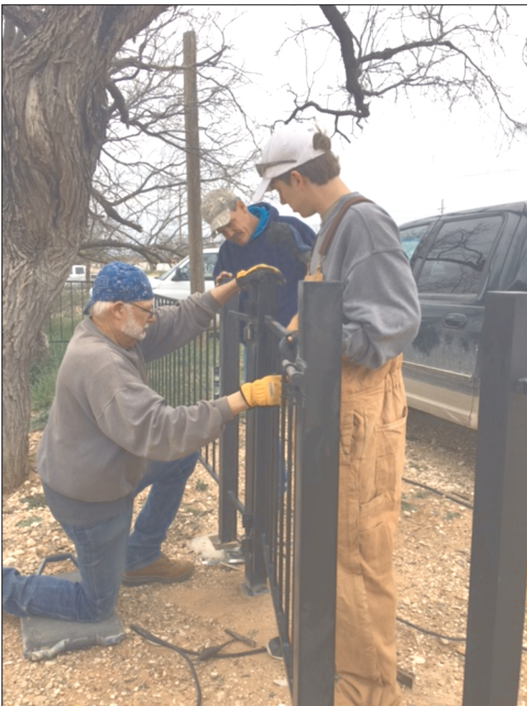
New Iron Fence! The hand forged iron fencing at the Old Coke County Jail, conceived and funded by Charles and Joy Millican Blake, is close to a reality with the hanging of the gates for the fence. Steve Clark, designer and welder (from left), Jeff McCrea, preservationist and contractor for Old Jail projects, and Ryan Jones, top hand in the fencing project are busy with the project.
