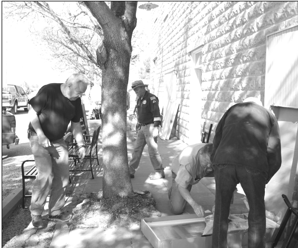
VP Volunteers! Members of Robert Lee's Vision with a Purpose work together to remodel the group's headquarters building on Austin Street in Robert Lee. Photo courtesy of Leta Caston.
