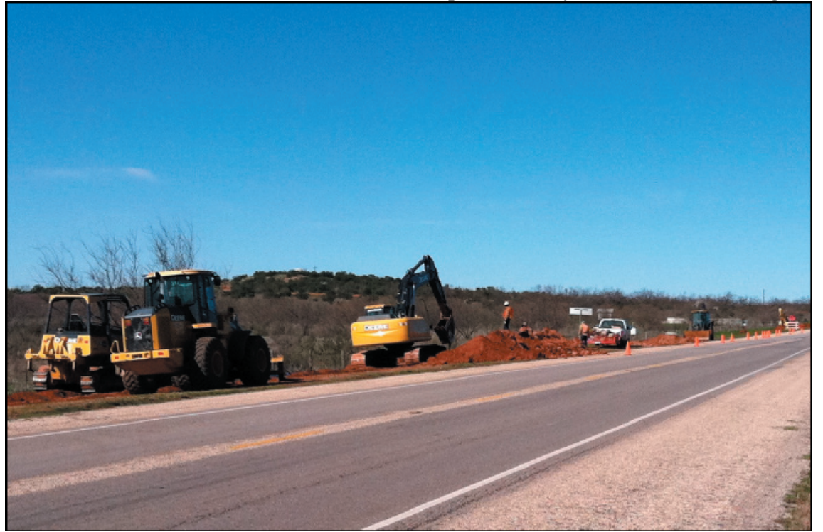
Pipeline Nears Completion! You can see in the photo above, taken Tuesday, March 20, that the two ends of the water pipeline running from Bronte to Robert Lee are only about 100 yards apart. The pumps will not arrive in Robert Lee until April 1, shoving the official completion date back to the middle of April. However, according to city officials, Robert Lee is in no danger of running out of water before the completion of the pipeline and pumping system.
