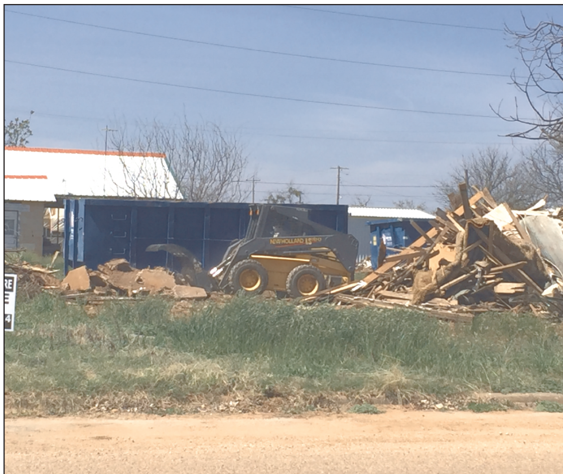
Bronte Demo! Bryan Swecker and Reese Braswell put in a couple of days of work last week and filled two large dumpsters removing the dilapidated house in Bronte on North Washington Street across from the water treatment plant. This is the first of many dilapidated houses Restoring Bronte Foundation and area volunteers have targeted for demolition in their quest to improve Bronte.
