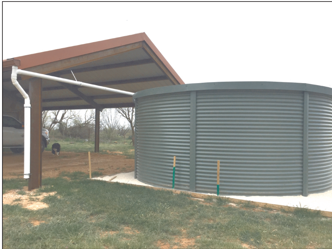
Catch System Example! Above is an example of a rainwater catch system using a metal roof, seamless gutters, first flush diverters and a metal tank with a plastic liner.
