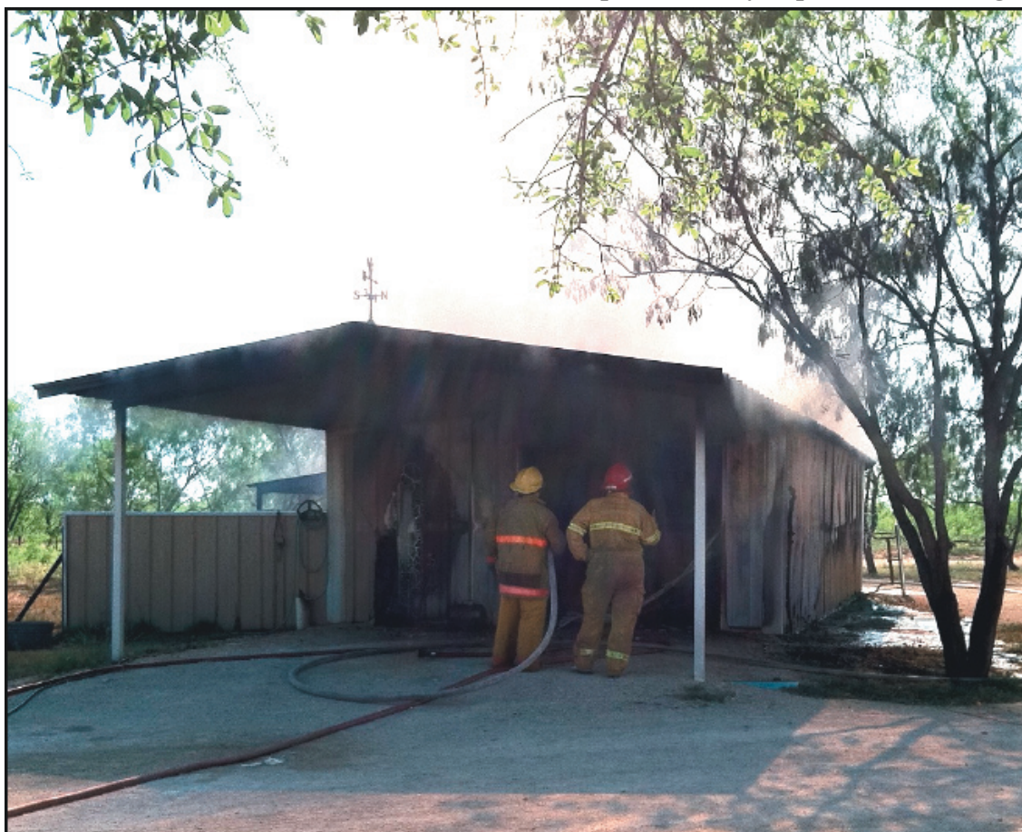
Barn Burns! Two members of the Bronte Volunteer Fire Department observe the damage caused by a fire Saturday afternoon, April 21, 2012. The structure is a barn owned by Jim Allen, local TPWD game warden. Although Allen was away, Sheriff's deputy, Brandon Neal was able to move the TPWD vehicle parked nearby.
