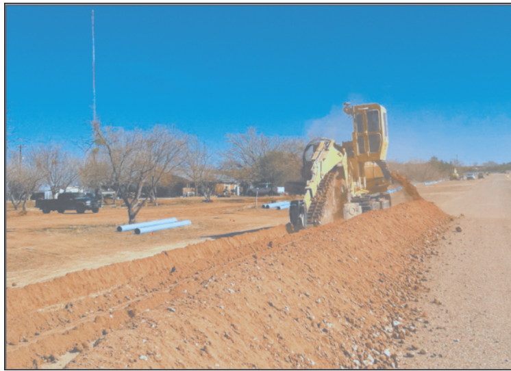
It's Begun! The construction of the trench for the water pipeline began Tuesday, January 17, 2012. The huge machine, along with the operator, were donated by Vermeer.
