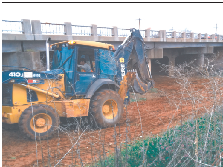
Water Pipeline! Roberts Construction of San Angelo began their section of the water pipeline at the Bronte water treatment plant. They are shown in late February 2012 covering up the section of pipe under the bridge over Highway 158 at the west edge of Bronte. Texas Water and Soil Company of San Angelo picked up where Robert Lee's volunteer requirement ended and headed west. They continued west to Double Barrel Road and then turned north to meet the Roberts Construction section at the intersection of Hwy 158 and Double Barrel Road.
