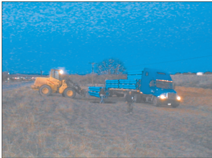
Miles of Pipe! The moon shines its last rays before the sun came up as Edwin Brosh of WEB Construction unloaded one of the trucks laden with the miles of pipe necessary for the water pipeline project.
