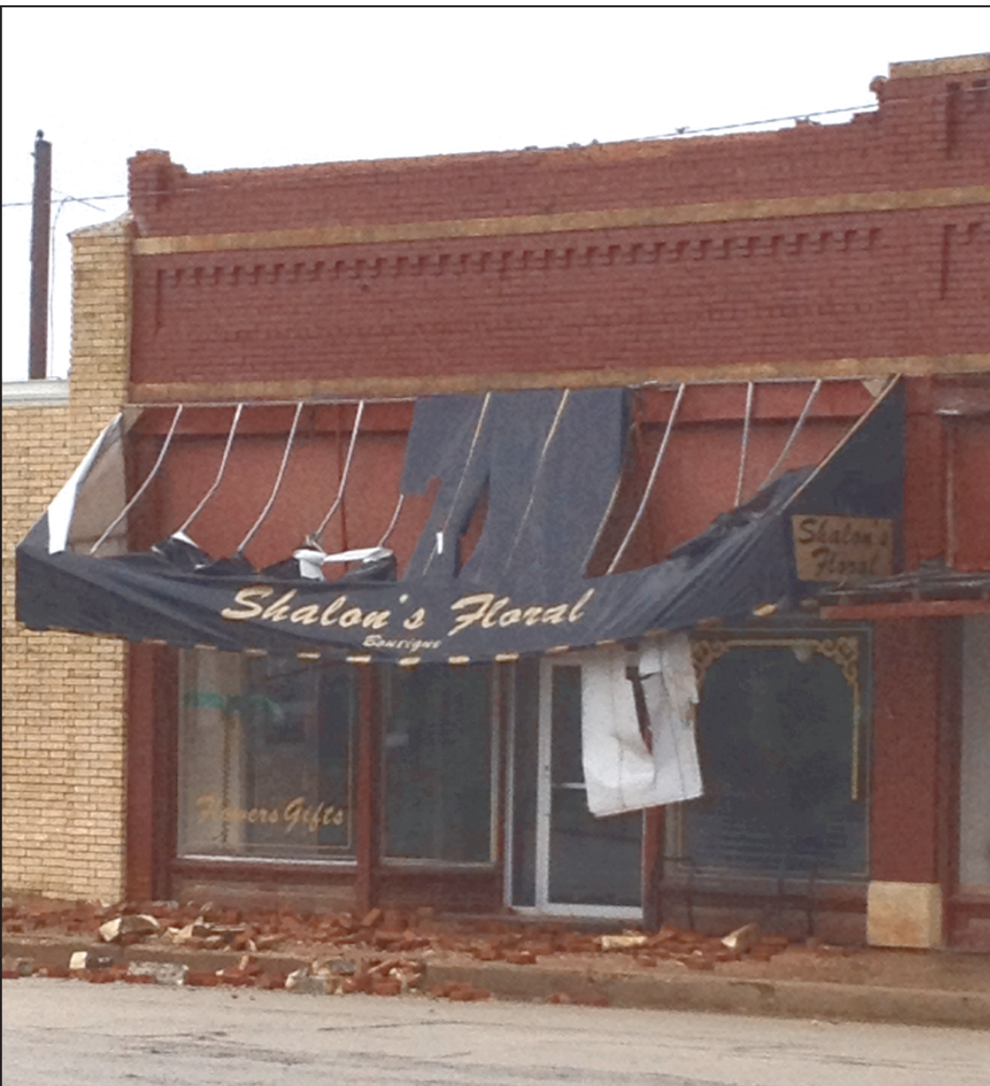
Storm Damage! Last week, another storm came through and proved to be the final straw for this awning in downtown Bronte.
