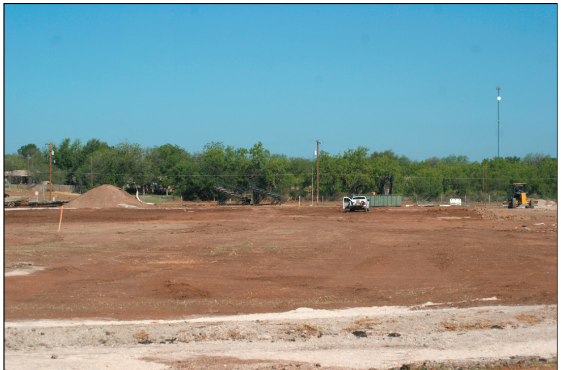
What a difference a couple of months make! The bottom photo is a look at the Robert Lee High School stadium the first of May. The top photo was taken last week. The new stadium should be completed by August 1st and the community can get a closer look when they attend the RLHS 2014 Project Graduation Hot Dog Supper the evening of August 15th. The first varsity game in the new stadium is set for 7:30 pm Friday night, August 30, 2013, between the Robert Lee Steers and the Longhorns of Meeteetse, Wyoming.
