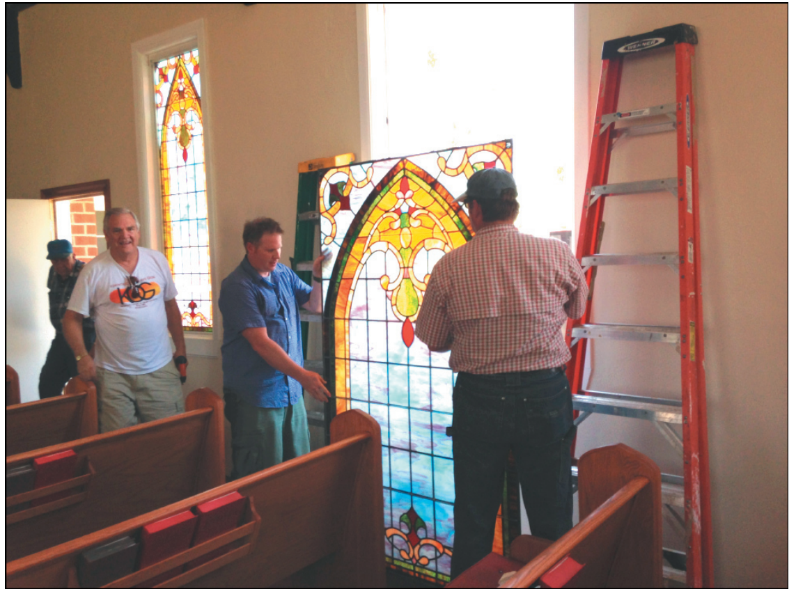
New Windows in Blackwell! Whitworth Stained Glass traveled to Blackwell last week to install the gorgeous new windows in the sanctuary of First United Methodist Church of Blackwell.
