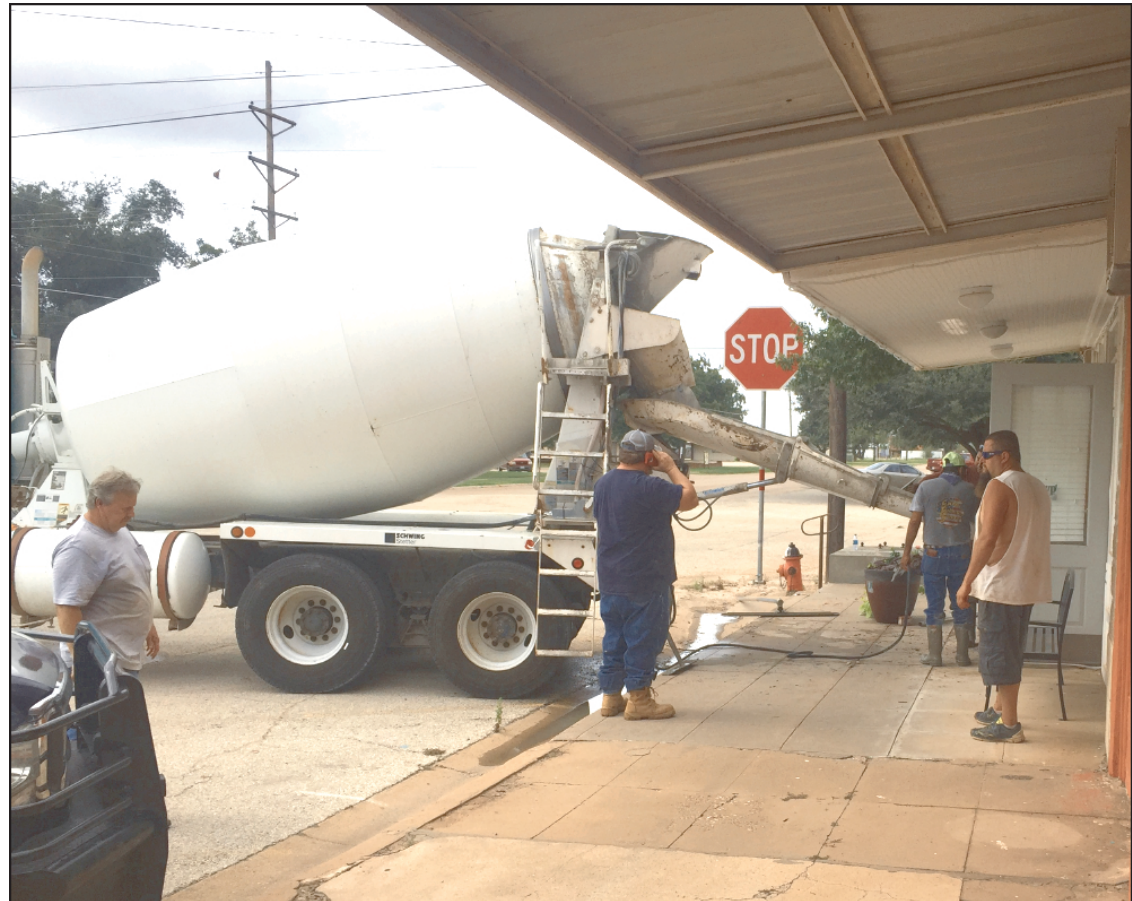
Vision Being Fulfilled! Robert Lee's Vision with a Purpose accepts a load of concrete during the remodel of their headquarters building on Austin in Robert Lee.
