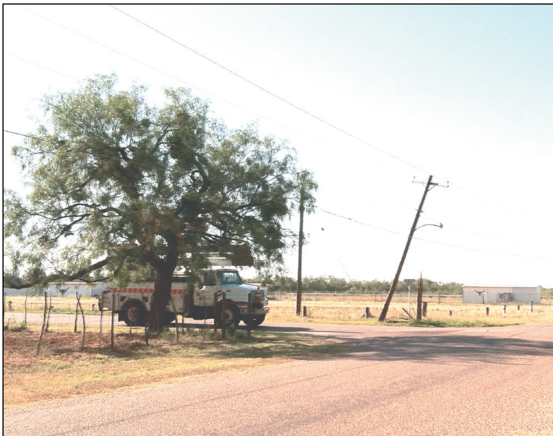
Broken Utility Pole! Someone broke this utility pole in the 600 block of South Jefferson in Bronte last Thursday morning, August 29, 2013, just after 8 am. Fortunately, no lines were on the ground.
